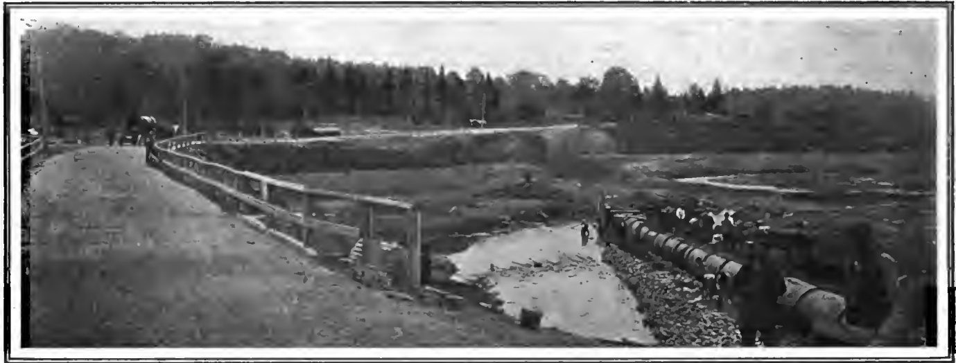
Fig. 1—View of the country where the Easton, Conn., pipe line is being laid, showing truck and some pipes on the road
